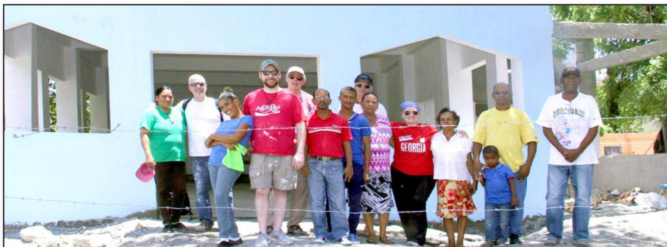
The St. Anne's missionaries with members of the Las Carreras community in front of the church building under construction.
